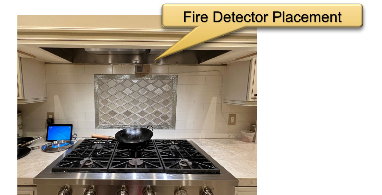
Fig 12. Kitchen with fire detector installed. (Photograph taken by Shanya Gill)
